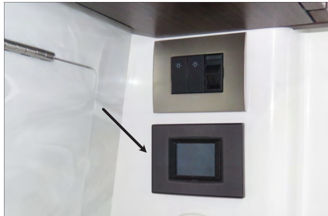
Air Conditioner Control Panel
