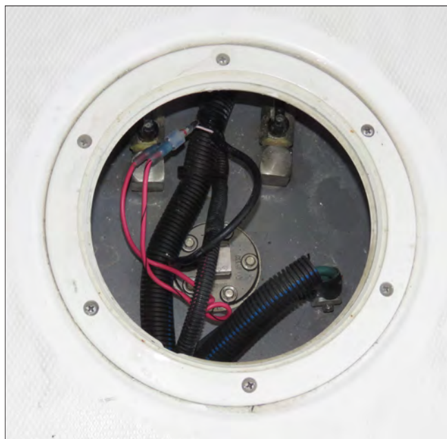
Typical Fuel Gauge Sender & Withdrawal Valves
