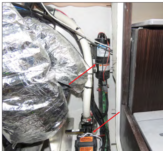
Overboard Macerator Discharge Pump & Electrically Activated Discharge Thru-Hull Valve In Forward Bilge
