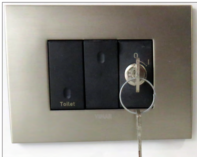
Toilet & Overboard Discharge Control Panel
