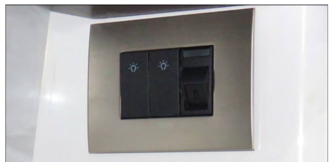
Cabin Light Switch Panel
