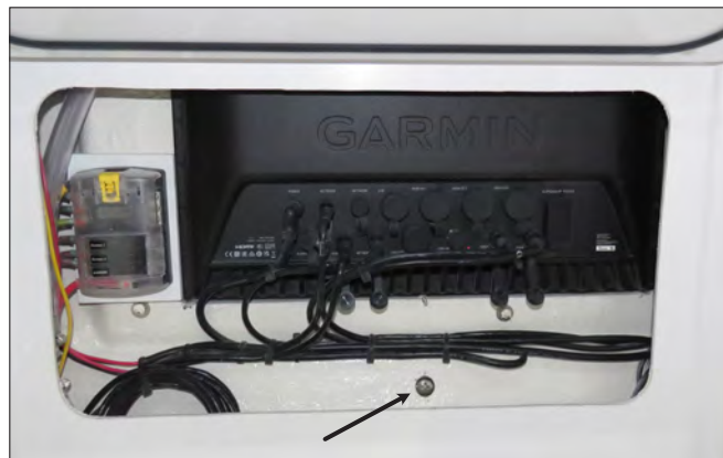
Helm Equipment Access & Bolts in Head Compartment
