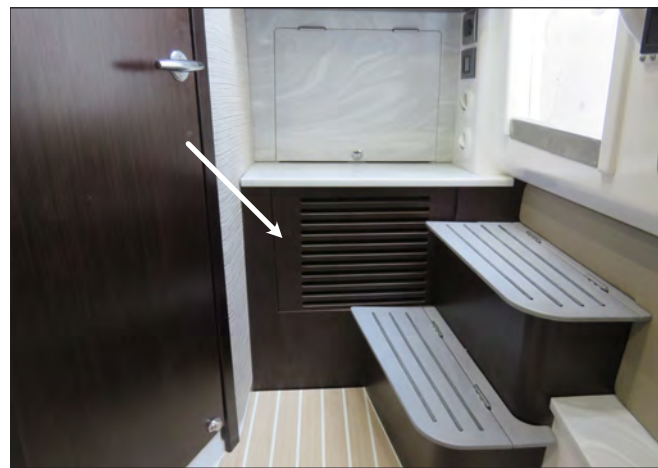
Air Conditioner Location Below Removable Countertop
