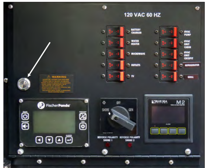
Bilge Blower Switch
