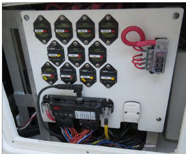
Digital Switch Control Module & Main Circuit Breakers
