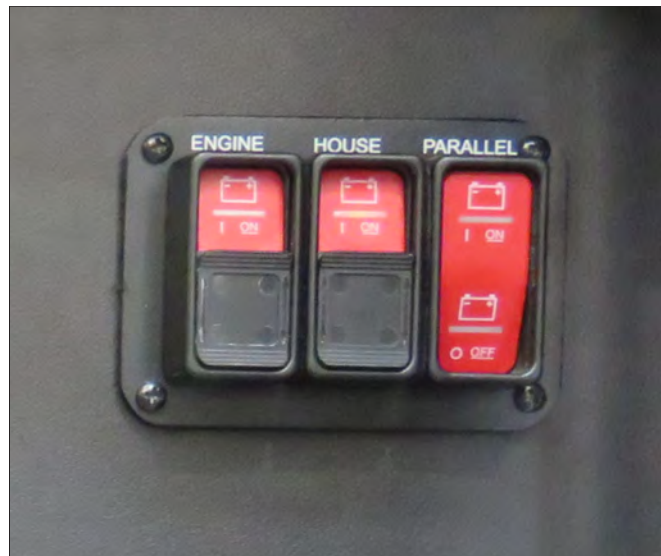
Remote Battery Switches On Cabin Electrical Panel
