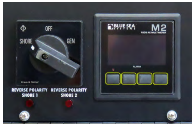
SHORE/OFF/GENERATOR Switch & Multimeter
