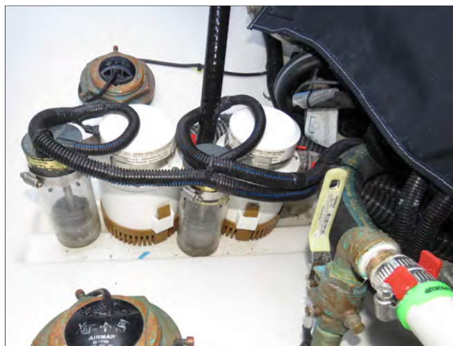
Aft Bilge Pumps & Automatic Switches
