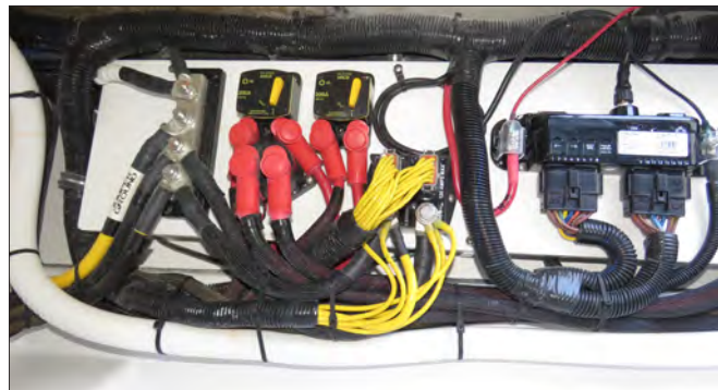
Yamaha Secondary Charge Lead Circuit Breakers & DCM In Aft Systems Compartment
