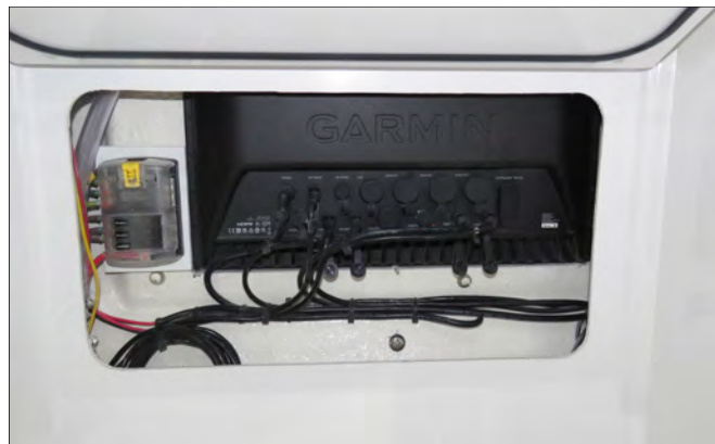
Electronics And Accessory Fuse Panel Behind Aft Head Compartment Bulkhead
