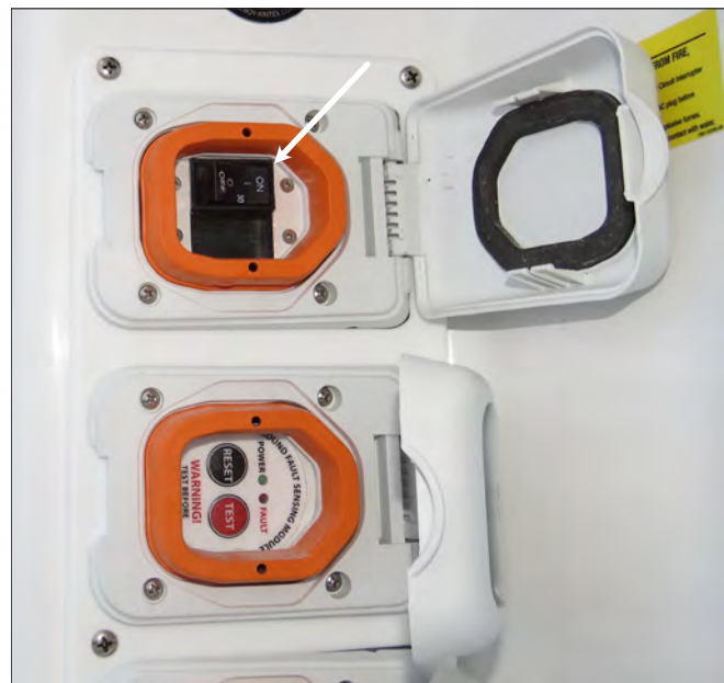
Inlet Main Circuit Breaker
