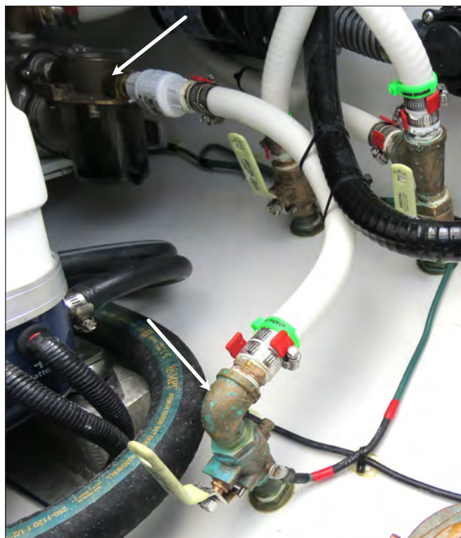
Air Conditioner Pump Strainer & Thru-Hull Valve
