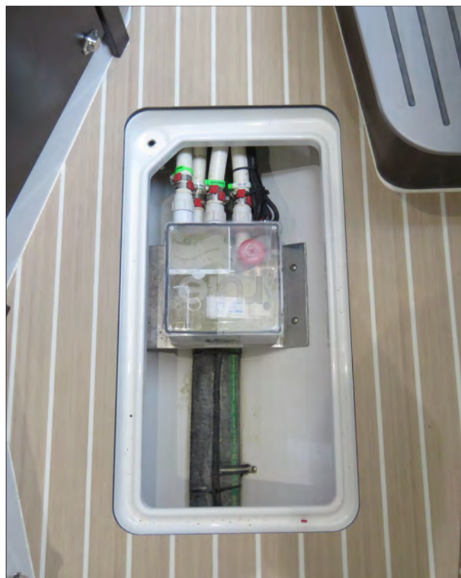
Shower & Cabin Drain Sump System
