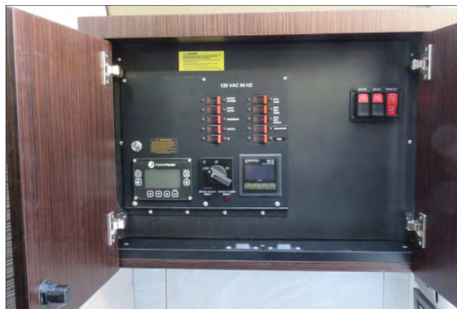
Hinged Electrical Panel In Aft Cabin Cabinet
