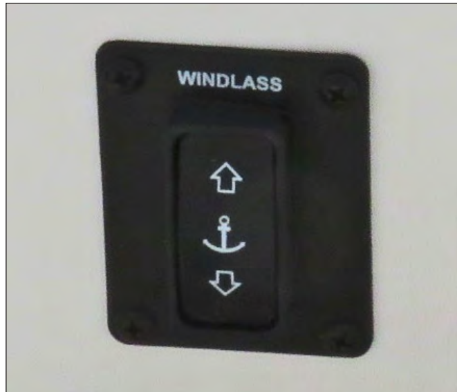
Windlass Switch In Windlass Compartment
