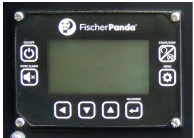
Generator Control Panel
