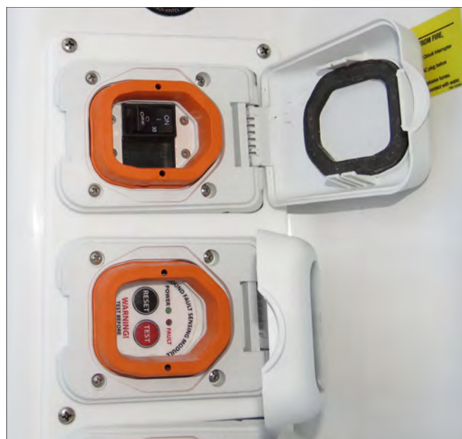
Typical ELCI Panel & Inlet Breaker
