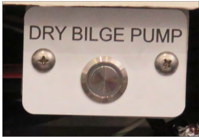
Dry Bilge Pump Switch
