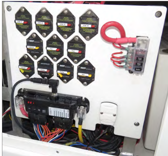
Main Circuit Breakers, DCM Module & Accessory Fuse Panel
