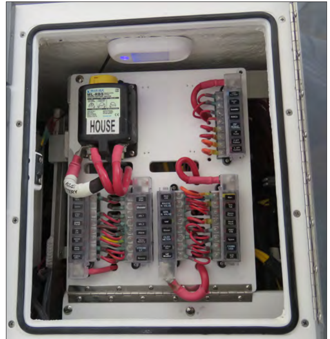
House Battery Switch & Fuse Panels
