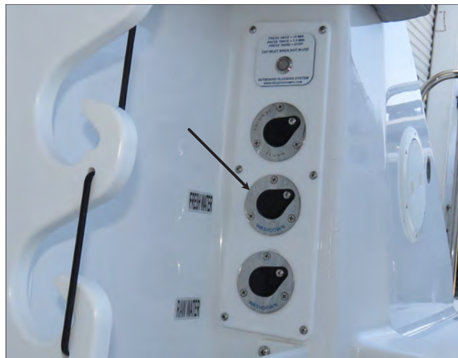
Cockpit Raw Water Washdown Connection
