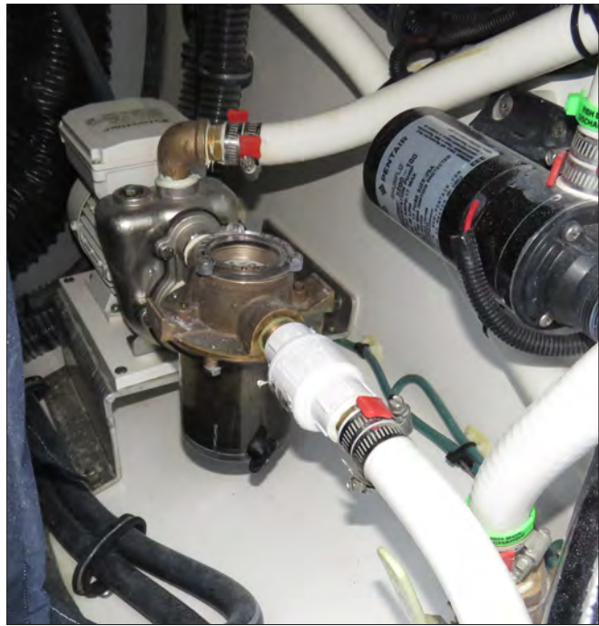
Air Conditioner Cooling Pump & Sea Strainer
