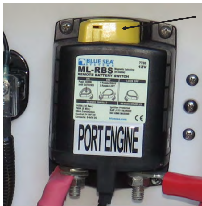
Engine Battery Switch & Manual Override
