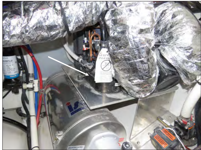
Air Conditioner Condensation Pan
