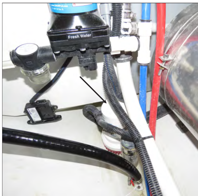
Forward Bilge Pump & Automatic Switch
