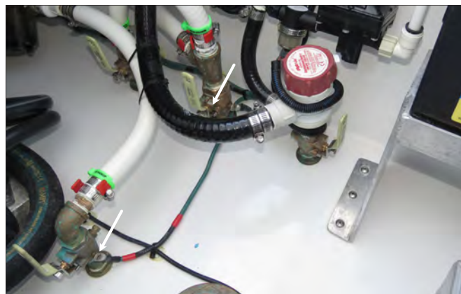
Typical Bonding Wires & Connections
