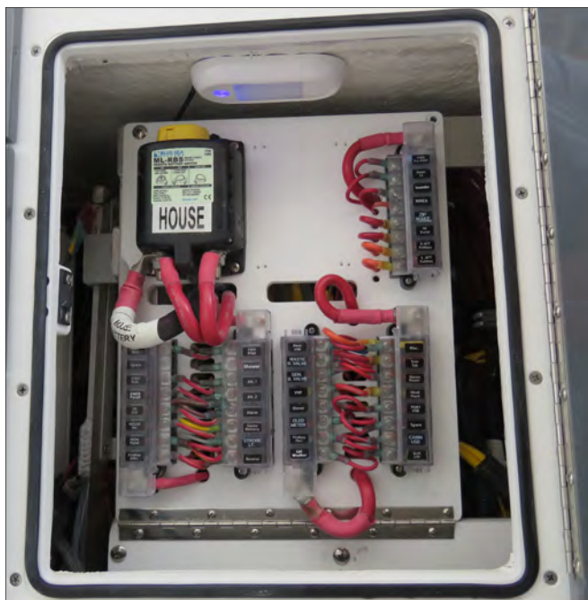
House Battery Switch
