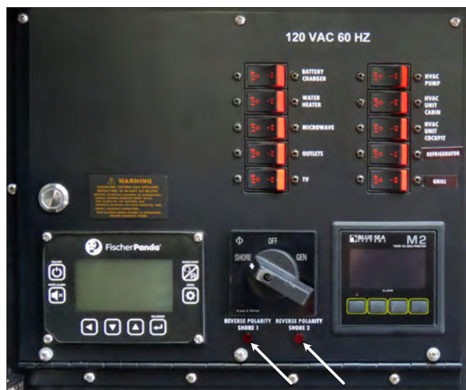
Cabin Electrical Panel Reverse Polarity Lights
