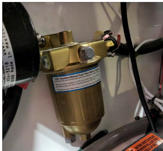
Generator Diesel Fuel Filter
