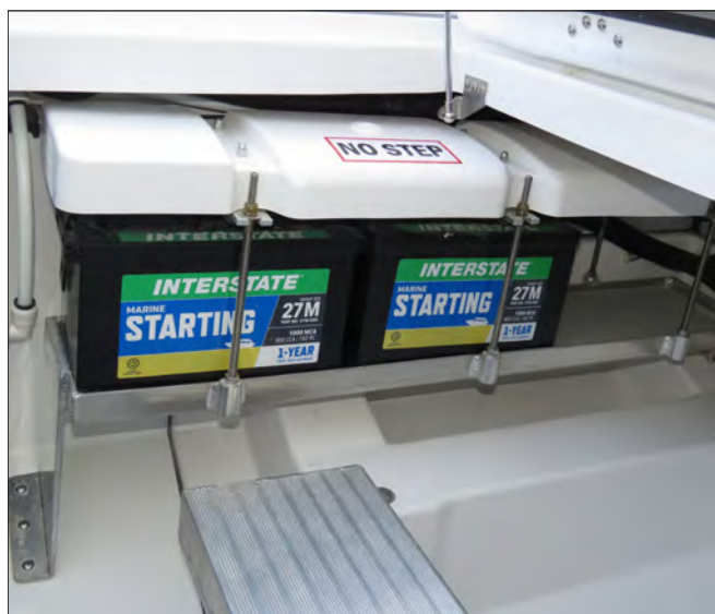
Engine Starting Batteries In Aft Systems Compartment
