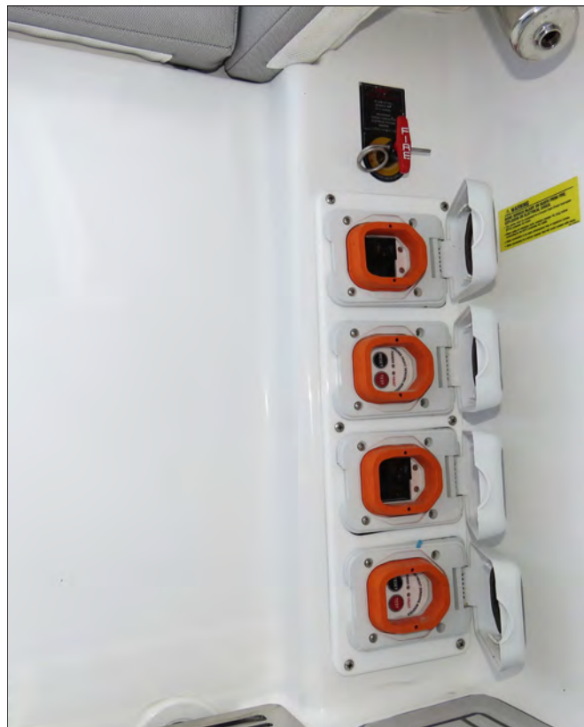
Typical Elci Panels & Inlet Breakers For Two Shore Power Inlet Plugs
